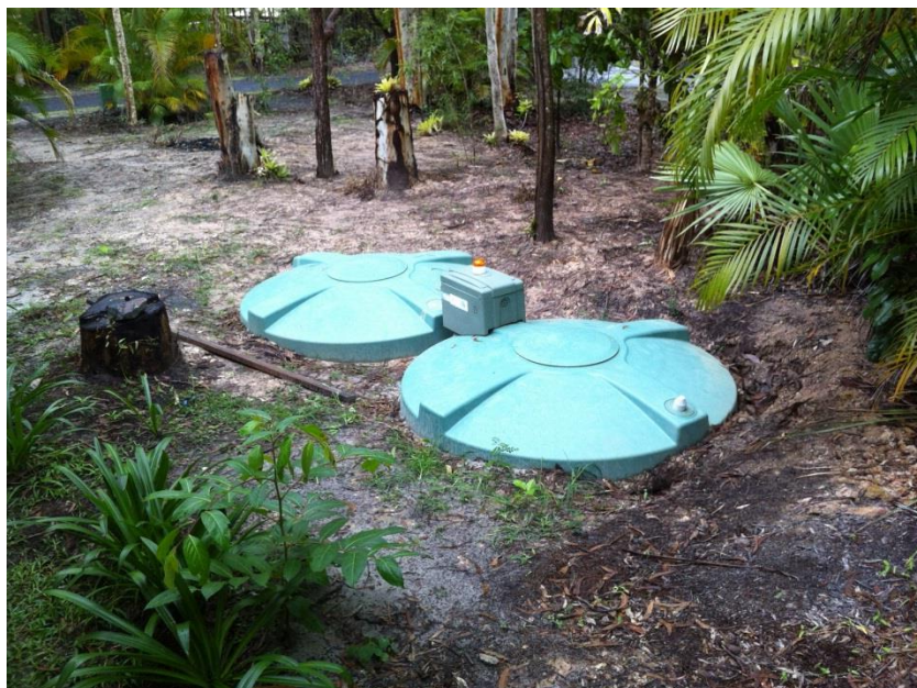
Figure 10 - A secondary treatment system serving a small dwelling
