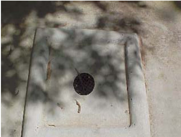
Figure 7.3 A bunded bin wash area in an unroofed bin enclosure, which is drained to sewer via a drain. Bund is no more than 100mm in height.
